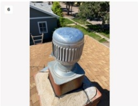
Hail damage to vent cap
